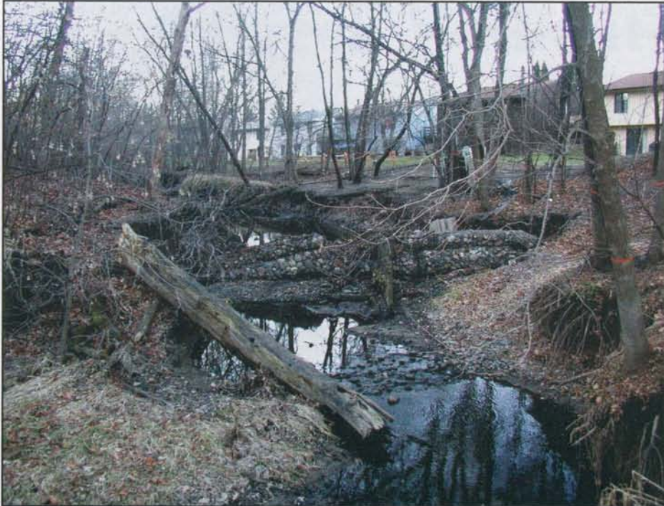
Before: The Pike Creek channel was a mess of previously attempted and failed stabilization structures, invasive vegetation, and low diversity degraded woodland.
