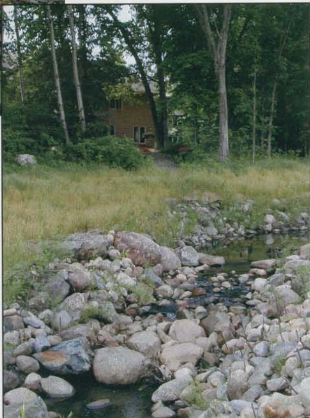
Top: Increased stormwater runoff in the watershed was causing Pike Creek to severely erode its banks, leading to property damage and poor water quality downstream. Inset: The same view as above shows the combination of hard armor and soft armor bioengineering techniques used to successfully stabilize the channel.
