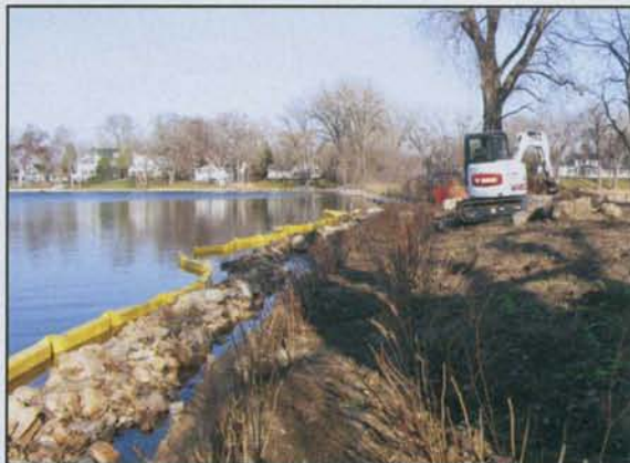
The Bobcat mini-backhoe is one example of a tracked vehicle that MacDonagh recommends. Unlike wheeled vehicles, tracked equipment won't cause severe soil compaction.
