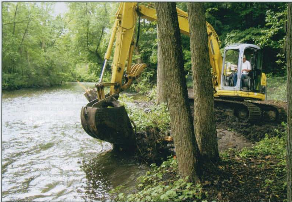
A backhoe is used to install a root wad at the shoreline. Not only do these create a habitat for fish, they are used to dissipate the water on the shoreline.
